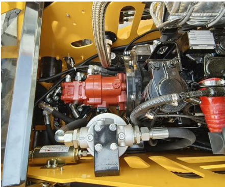
Two piston pumps and a gear pump
